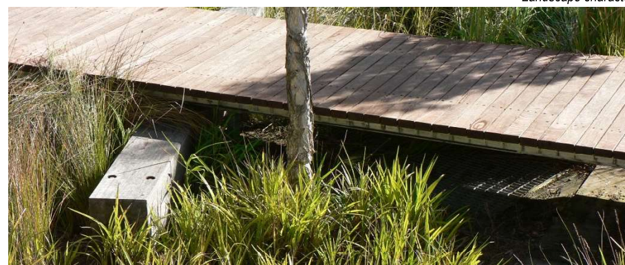
Planted drainage channels
